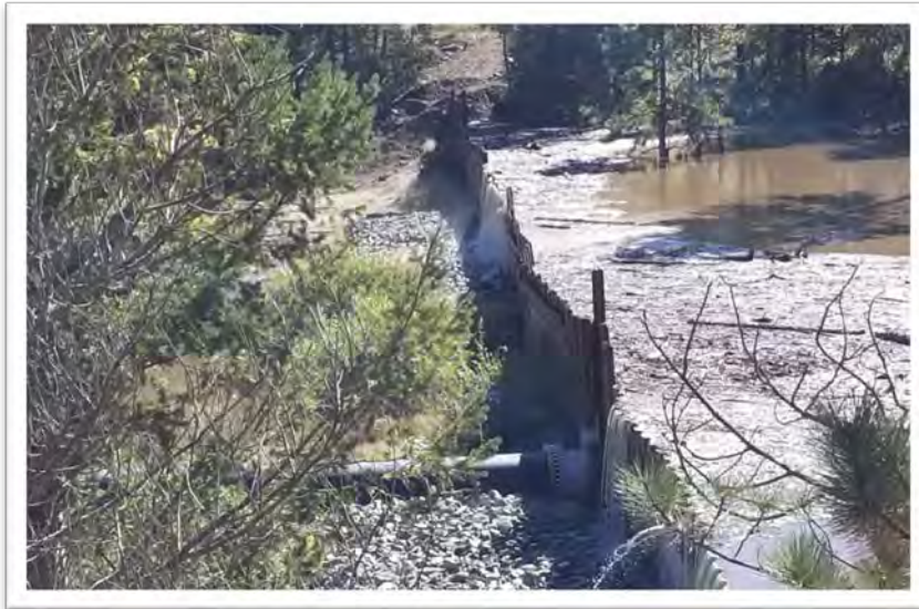
Coffer Dam Overtopped During Unordinary Storm Event
