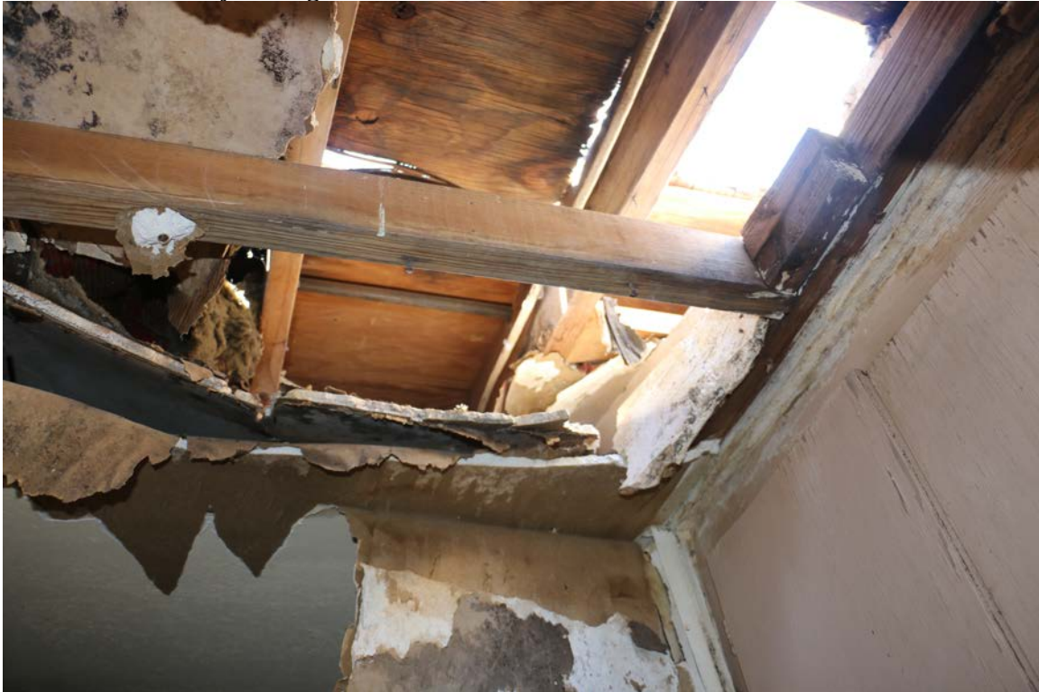
Photo #151 hallway ceiling to bathroom
