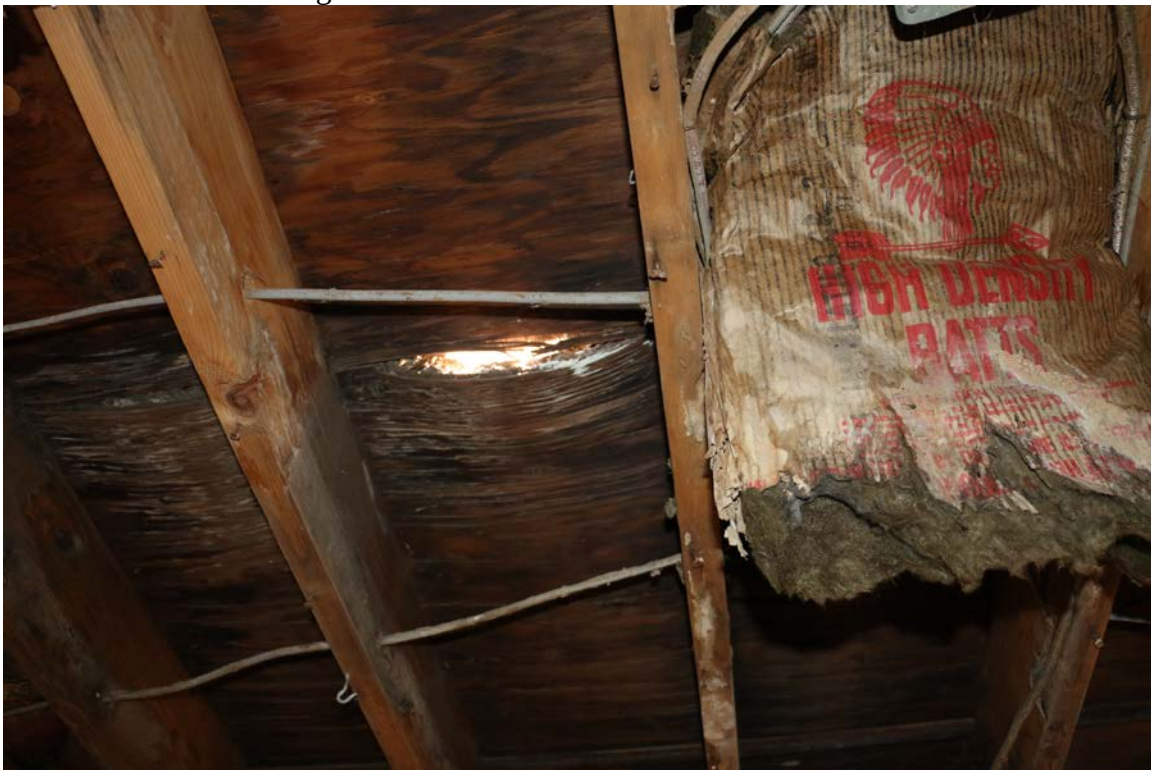
Photo #95 kitchen ceiling
