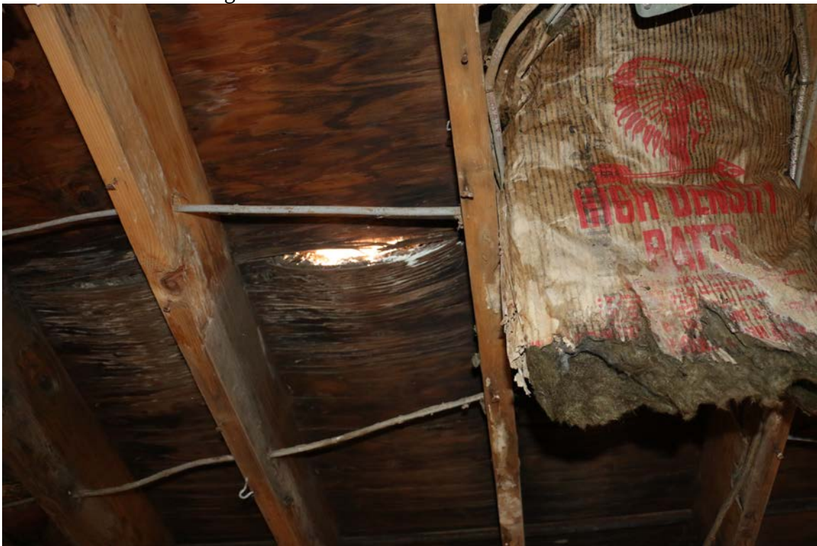
Photo #95 kitchen ceiling
