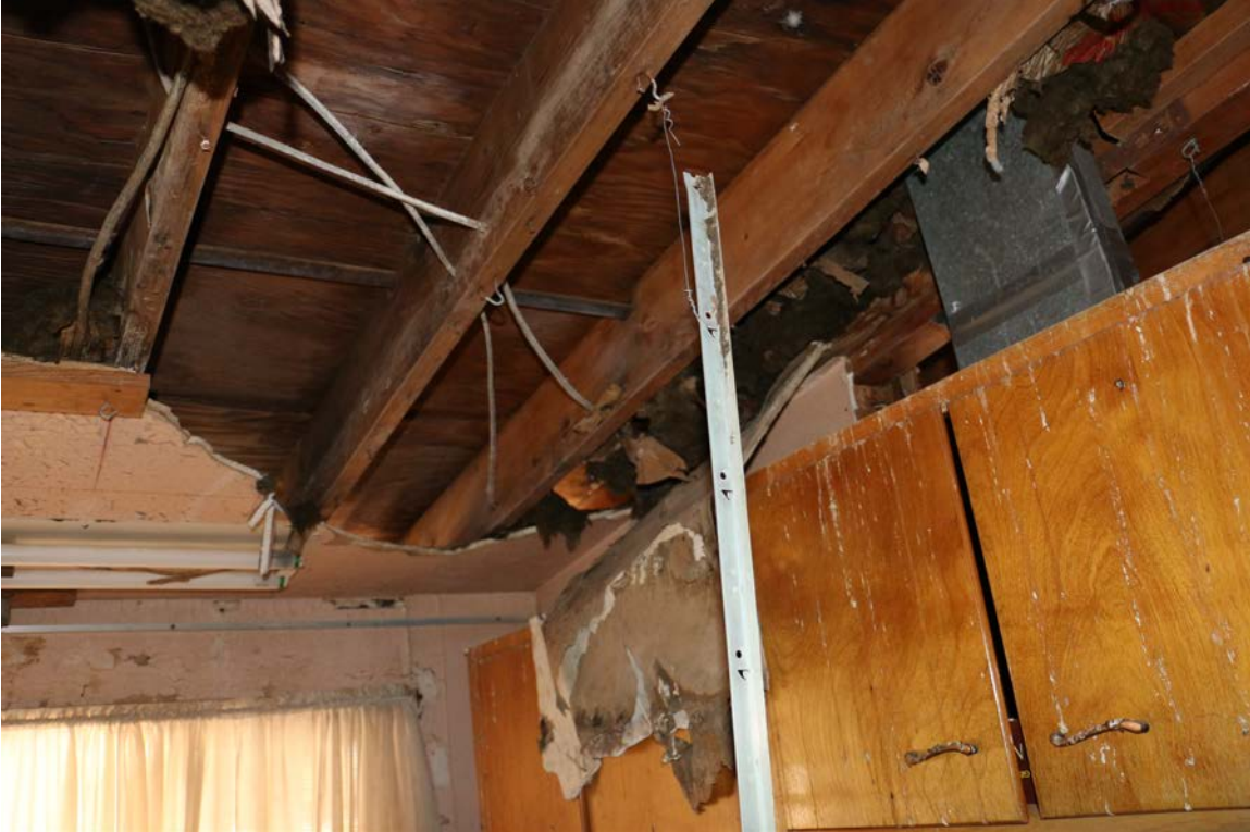
Photo #96 kitchen ceiling
