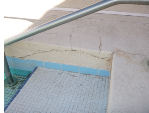
Pool structure cracking
