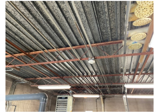
Mechanical room roof corrosion
