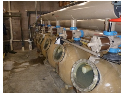
Swimming Pool Filtration
