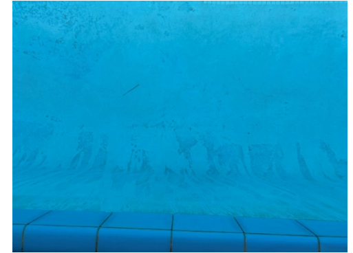
Pool surface staining/etching
