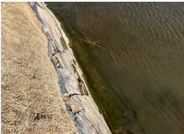
Exposed pond liner.
