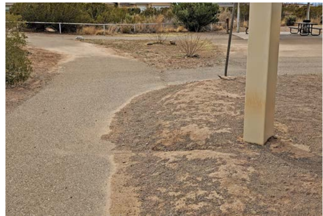
Sedimentation washing onto walkway.
