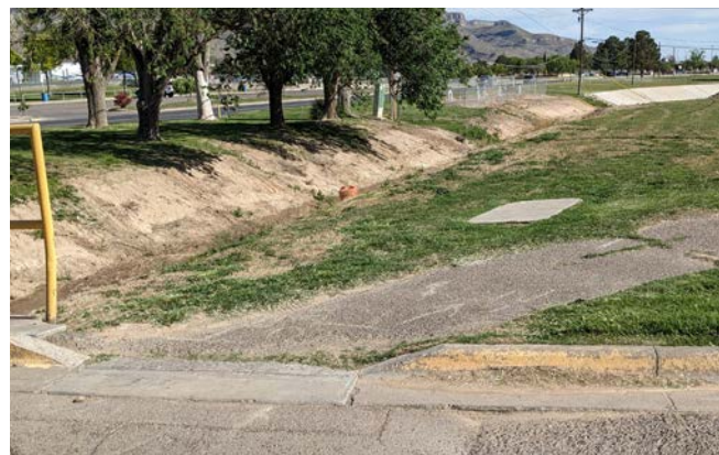
Non-accessible access at Mountain View Avenue.
