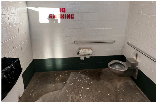
Restrooms do not meet accessibility standards.
