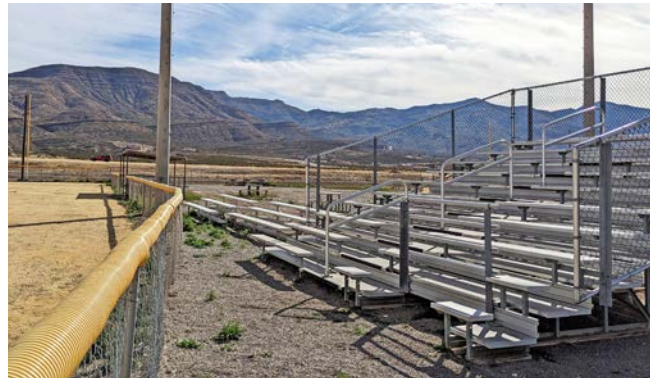
Bleachers with ADA areas but no ADA pathway.
