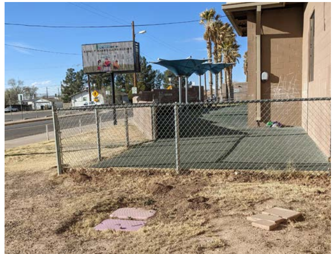
Patchy turf grass, sunken irrigation boxes, and trip hazards.
