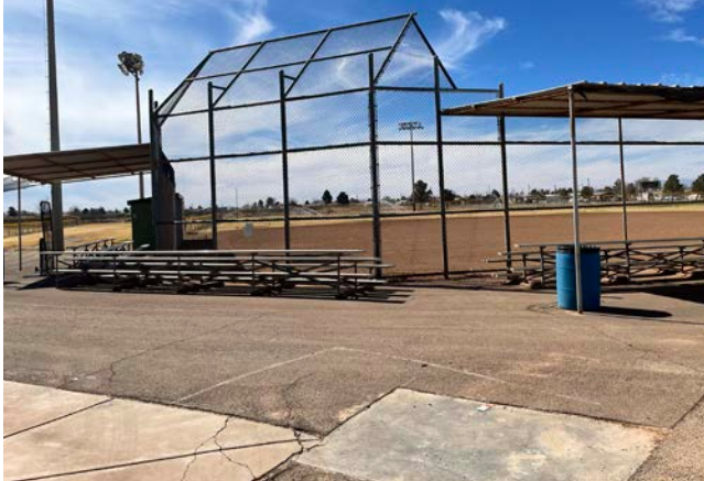
Cracked paving behind bleachers.
