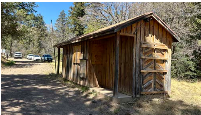
Dilapidated entry gate shack at West Lake Campground.
