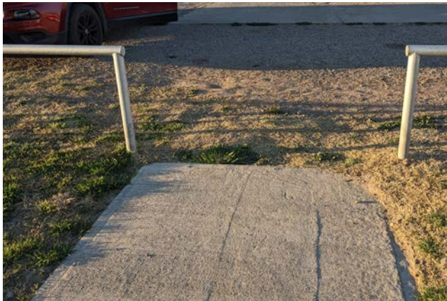
Handicapped ramp at parking lot does not meet accessibility standards and there is no designated accessible parking.
