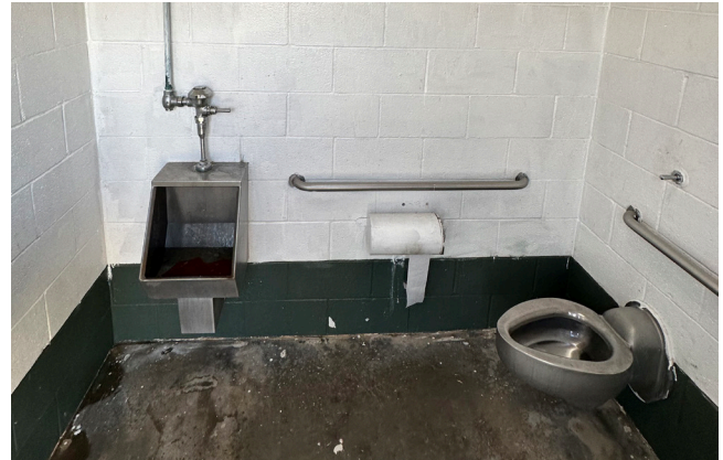
West restroom interior does not meet ADA standards.
