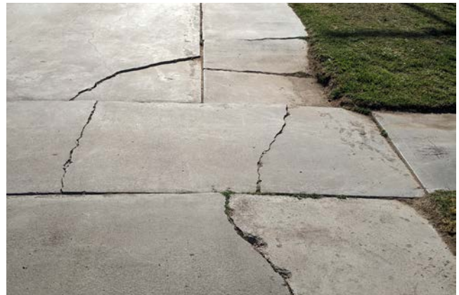
Cracked and heaving sidewalks.
