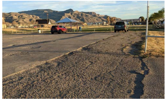
Parking shared with the Oregon Soccer fields is deteriorated.
