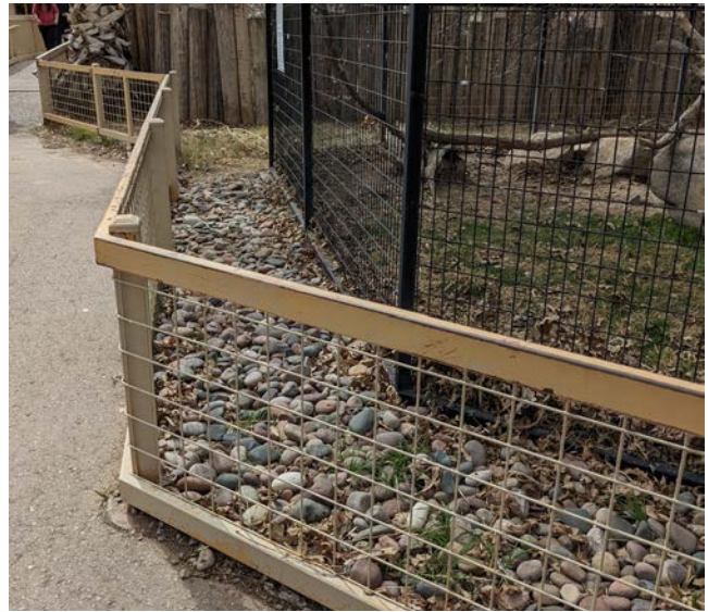
Landscape needs to be installed between the two barrier fences.
