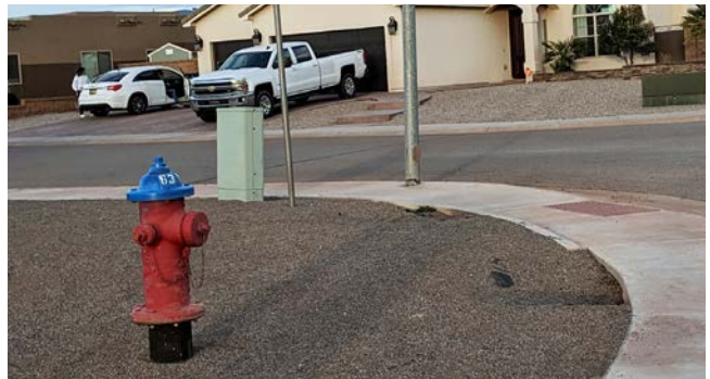
Drainage is undermining handicapped ramp.
