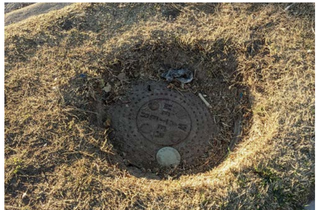
Thatch build-up around utility cans cause tripping hazard.
