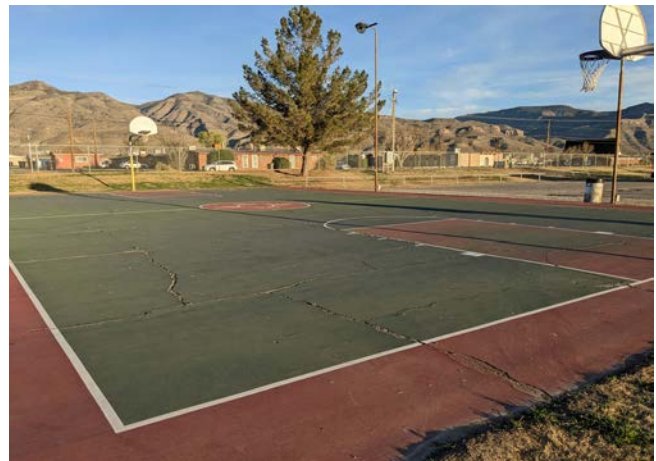
Basketball court surface is badly cracked.
