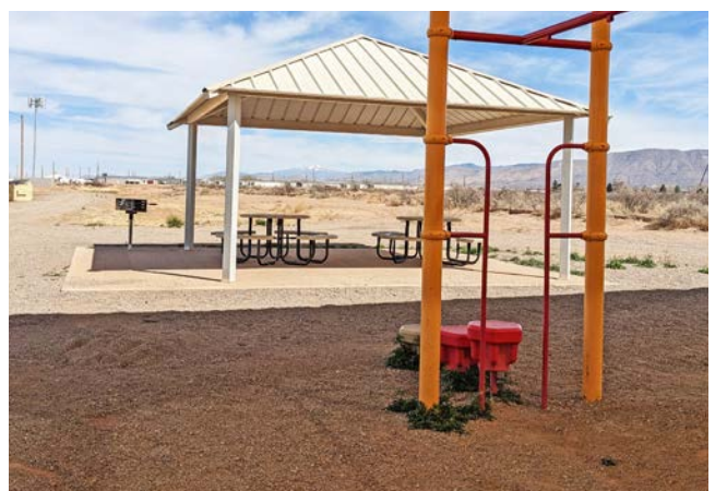
Play equipment with weeds growing in surfacing.
