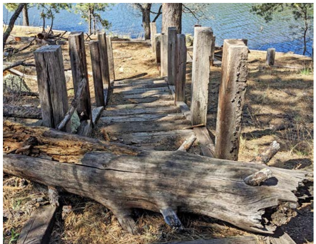
Missing handrails at the stairway and access blocked by fallen tree stump.
