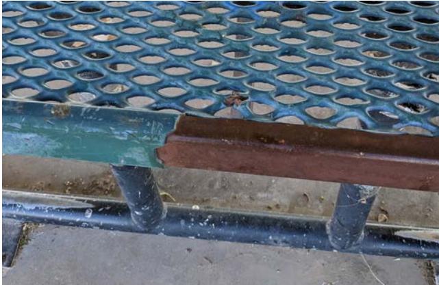
Exposed metal on picnic tables.
