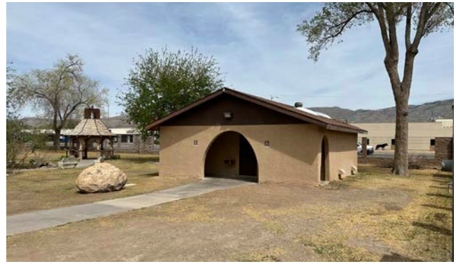
All restrooms need to be updated to meet ADA standards.
