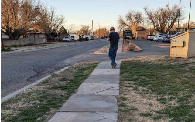
Cracked and heaving sidewalk.
