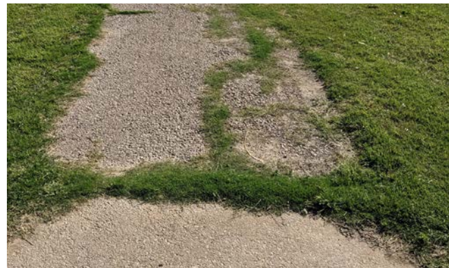
Asphalt trail with cracks and intrusion of grass.
