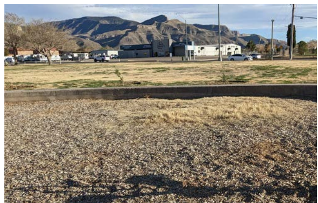
Turf is encroaching on playground surface.
