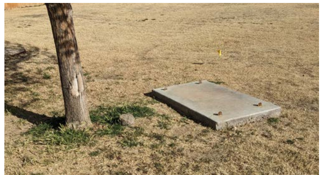
Damaged tree trunk and concrete pad with protruding bolts and missing a bench.
