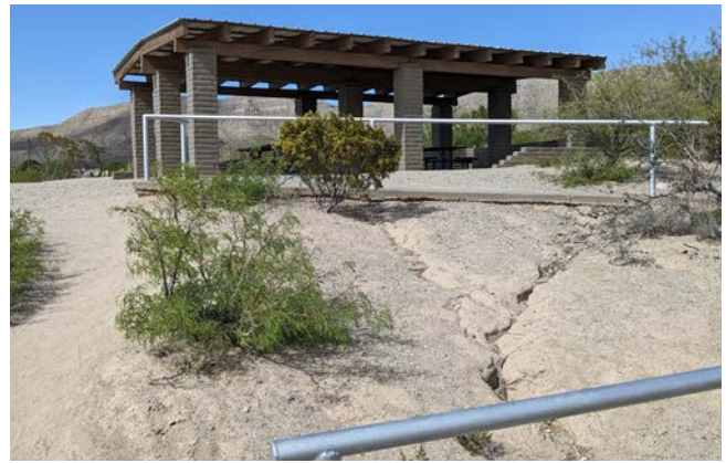
Erosion from drainage is comprising the ramp.
