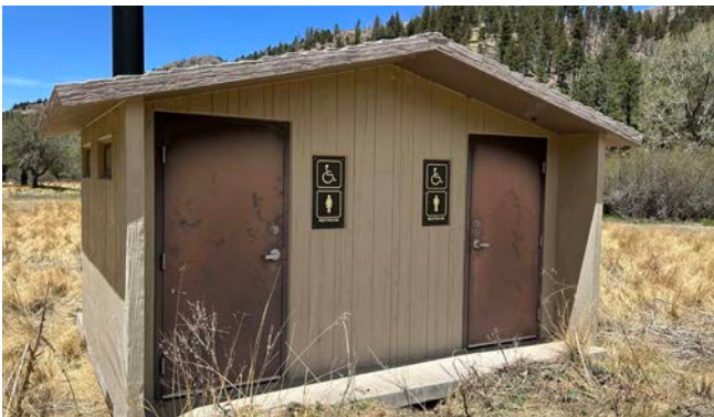
Damaged restroom building at Blue Hole/Apple Orchard.
