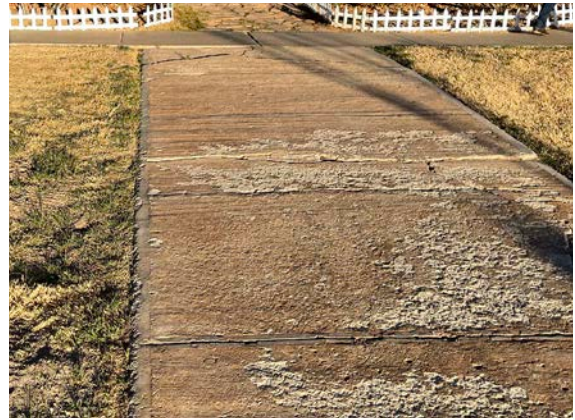
Spalling concrete sidewalk.
