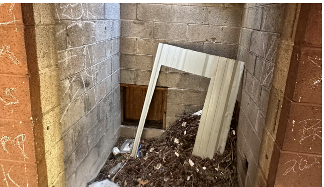
Deteriorated outhouse near the Blue Hole pond.
