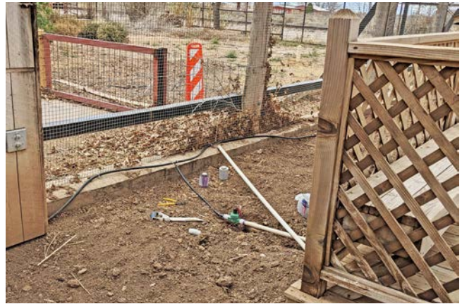
Aviary irrigation system needs to be upgraded.
