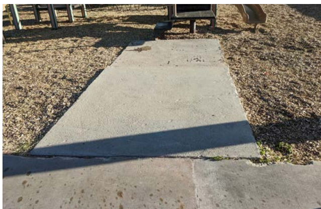
Deteriorated concrete path to play equipment.
