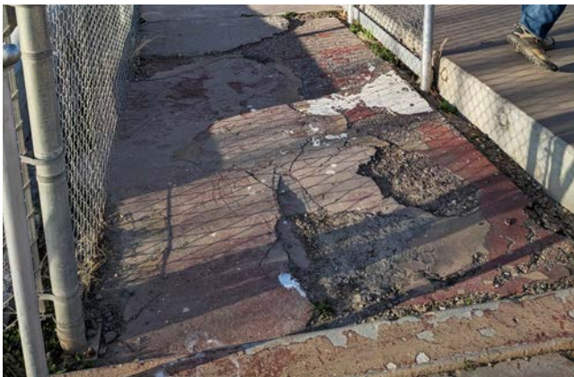
Cracked and spalling concrete.
