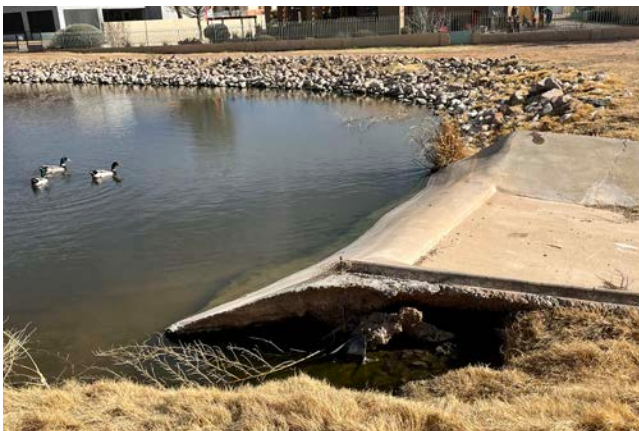
Soil underneath concrete ramp between ponds is washed out.
