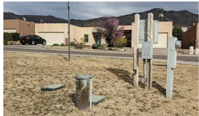
Irrigation well, controller, and valve.
