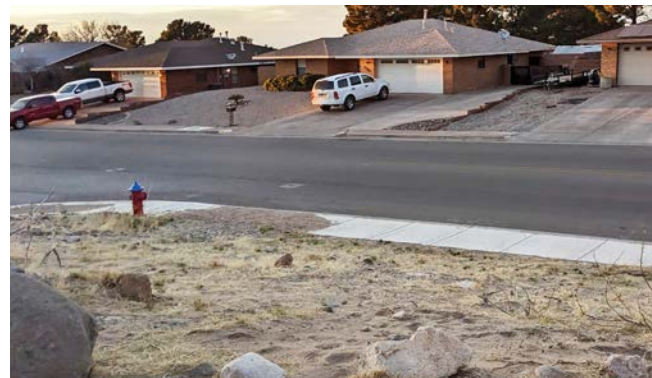
Sediment washing downslope across the public sidewalk.
