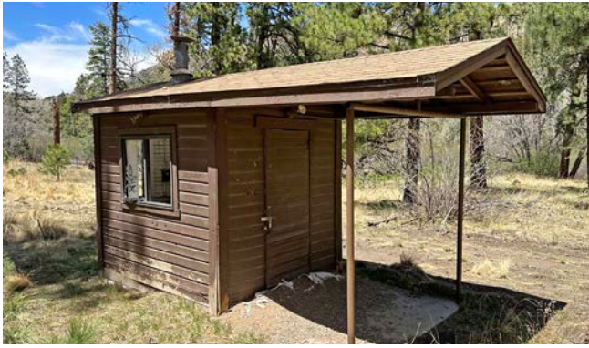
Dilapidated entry gate shack at Blue Hole/Apple Orchard.
