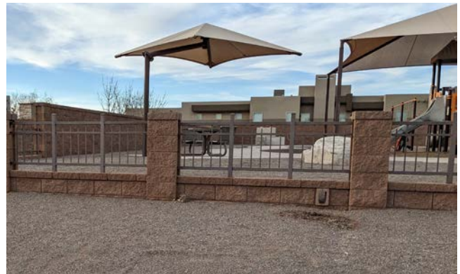
The drainage from the play area is impacting the adjacent gravel surfaced slope.
