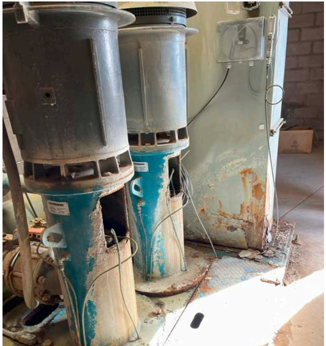
Booster pump house with corroded equipment.
