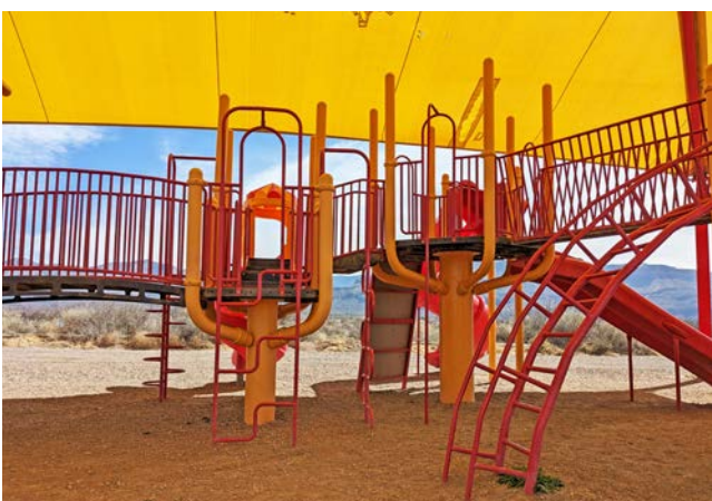
Shade cloth has patched holes and weeds are growing through the playground surfacing.
