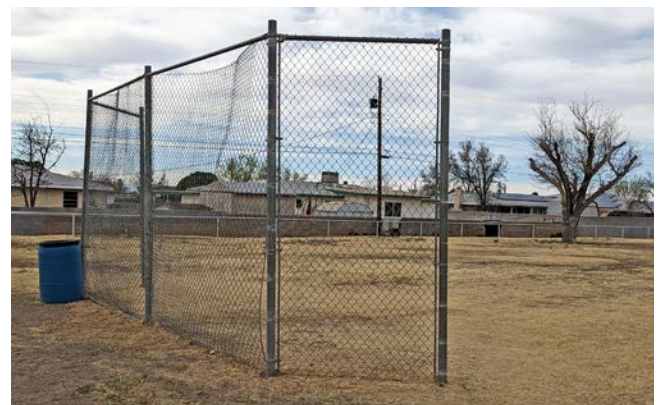
Bent and damaged backstop mesh fence.
