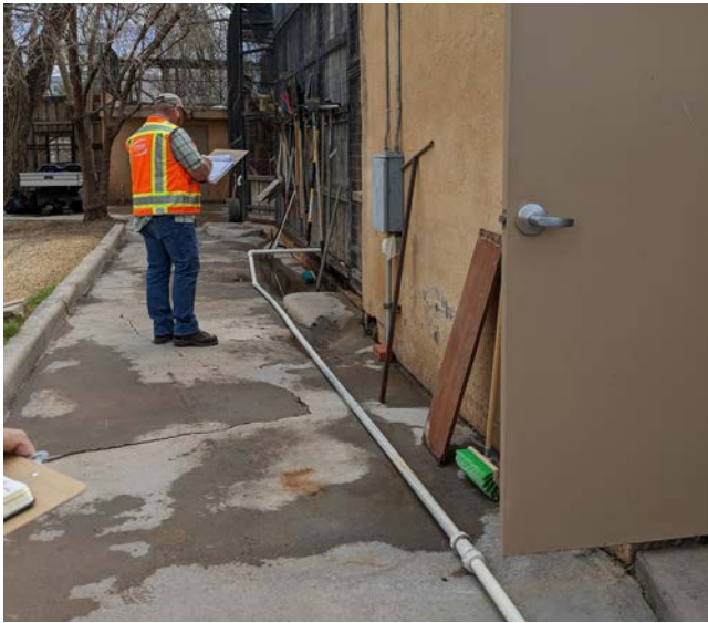
Drainage issues and the subfloor drainage system behind the otter exhibit.
