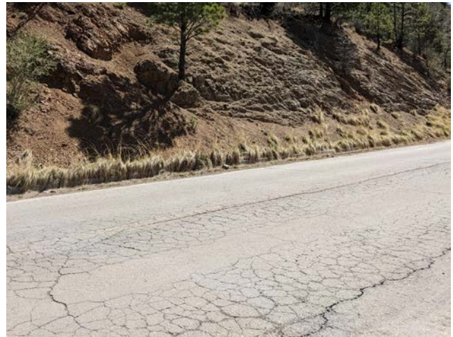
Road has severe cracking and is deteriorating.
