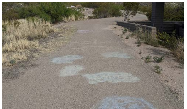
Deteriorated trail surface and landscape encroachment.
