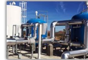
Plumbing – Controls, Conditioners, Pumps, Manifolds, Fixtures
