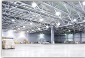
Facility & Exterior LED Lighting
