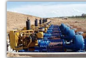
Irrigation Systems – Controllers, Pipes, Pumps, Valves, Emitters
