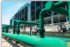
Boilers, Chillers, Cooling Towers, Air Handlers
