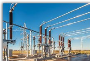
Electrical Distribution, Storage, Optimization & Generation
